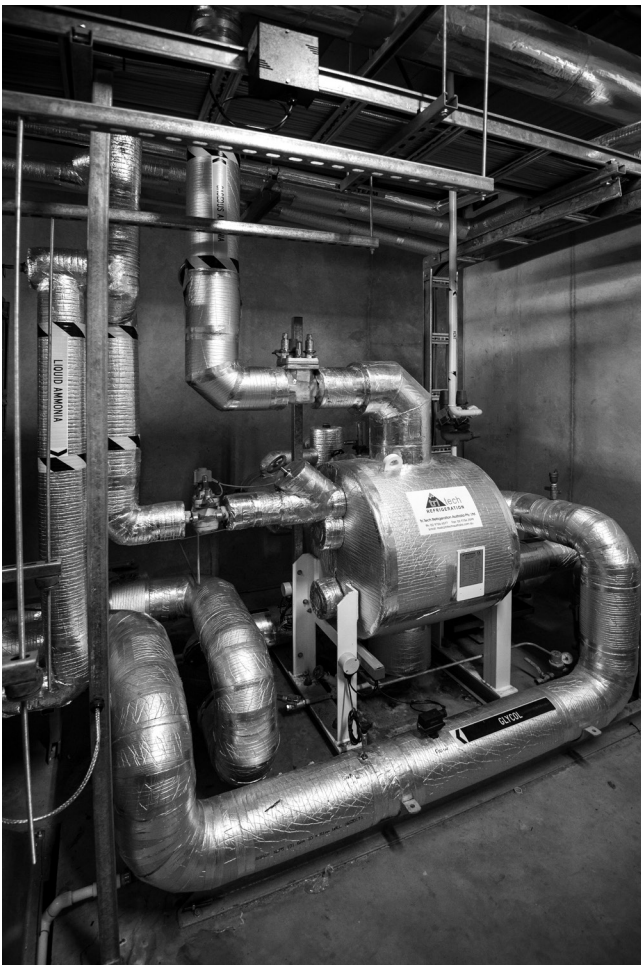
A 250 KW pumped glycol skid with Vahterus Combined PSHE in service at Zammit factory in Sydney, Australia.
