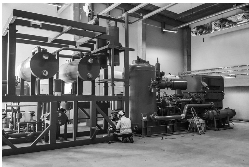
E.ON installation of four GEA heat pumps next to the sewage treatment and waste incinerator plant in Malmö, Sweden. The heat-pump system draws nearly 30 MW of heat from the sewage water Malmö's harbour area.
