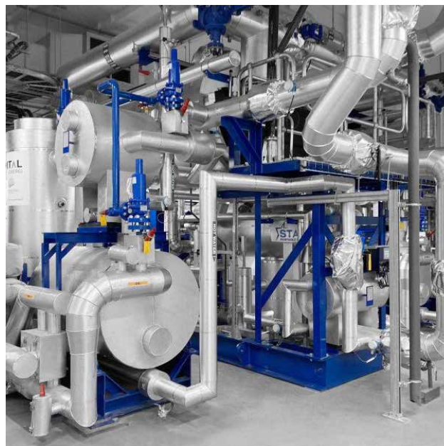
Star Heat Pump in the Energy Centre at Queens Quay. CO 2 savings compared to gas are 80% and improving.
